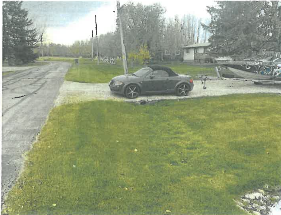
C209 – MISSING RIP RAP AND BURIED
