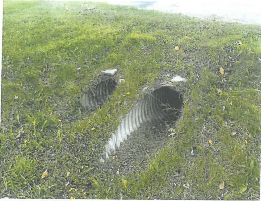
C206 & 207 – UNDERSIZED FOR ROAD CROSSING AND MINIMAL COVER
