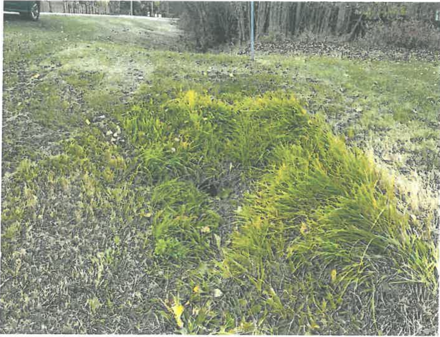
C103 – MISSING RIP RAP AND REQUIRES DITCH GRADING
