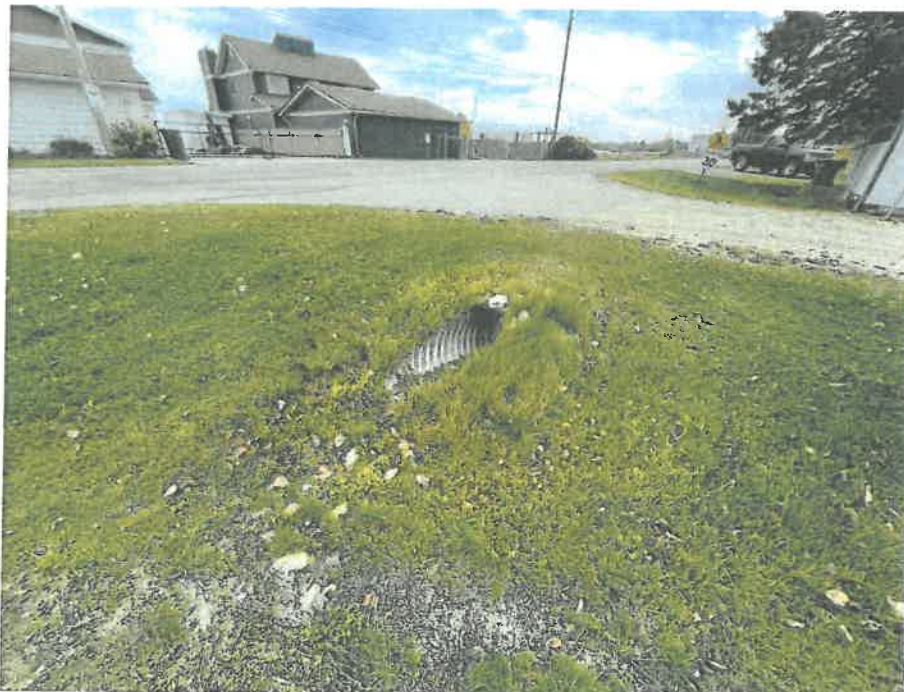
C149 – MISSING RIP RAP AND UNDERSIZED FOR ROAD CROSSING
