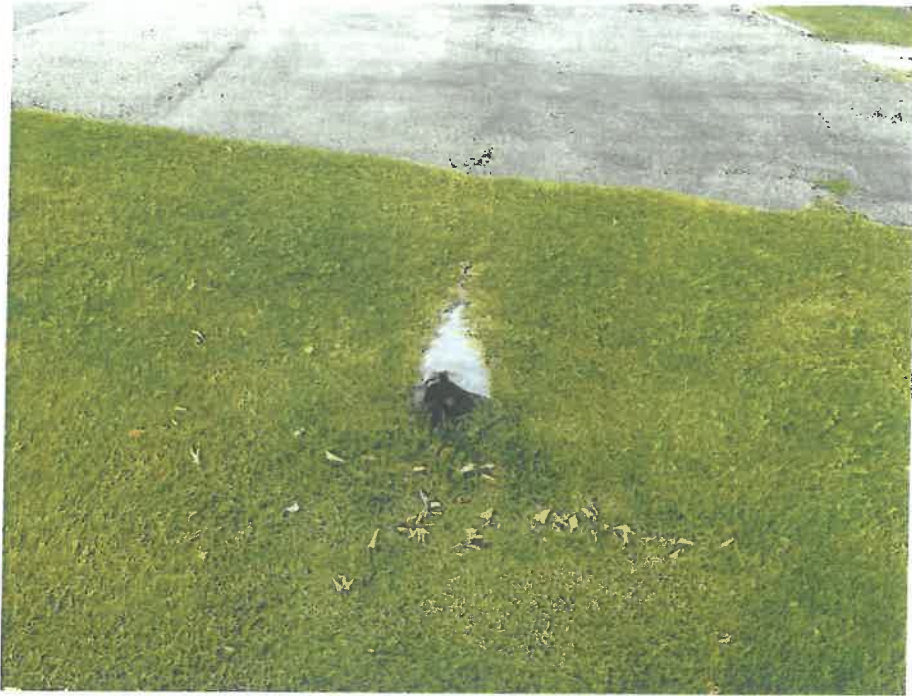
C193 – FLATTENED AND UNDERSIZED
