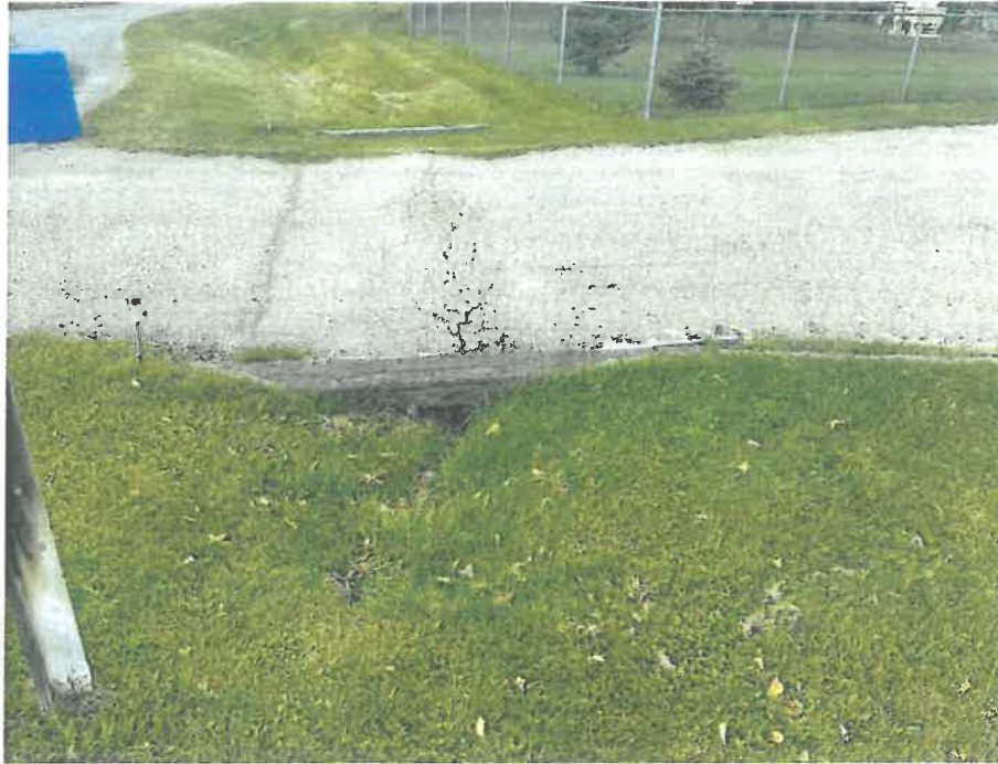
C191 – HEAVING AND UNDERSIZED
