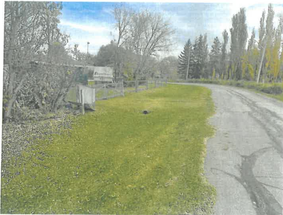
C205 – MISSING RIP RAP
