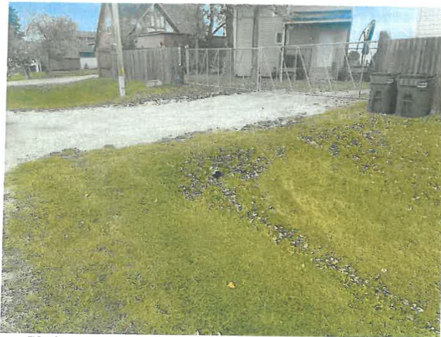
C152 – MISSING RIP RAP AND HIGHER THAN DITCH
