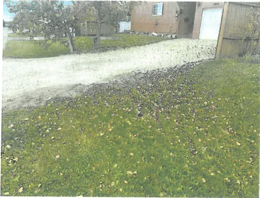
C153 – MISSING RIP RAP AND HIGHER THAN DITCH
