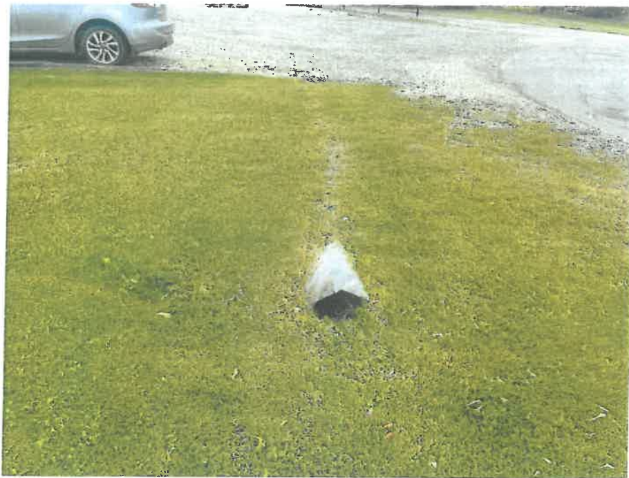
C192 – FLATTENED AND UNDERSIZED
